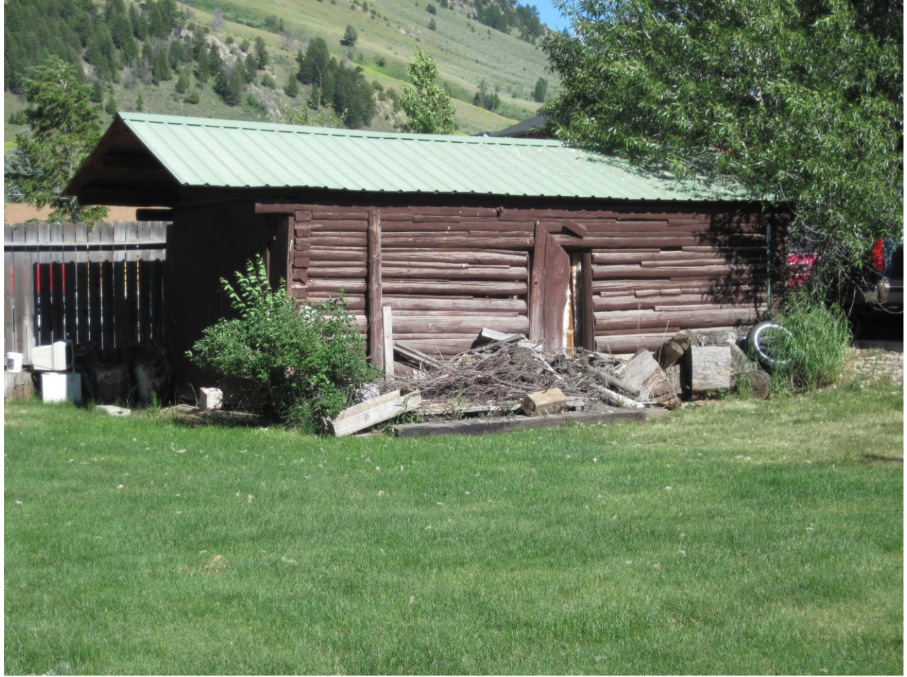
First Baptist Church of Jackson Hole Parsonage, Garage, West and North Elevations, Longfield, 2009
